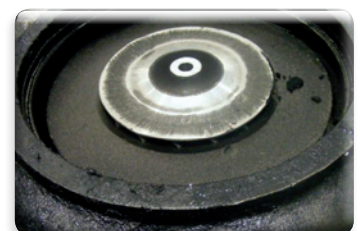
Compressor end oil leakage
