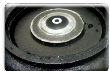
Compressor end oil leakage
